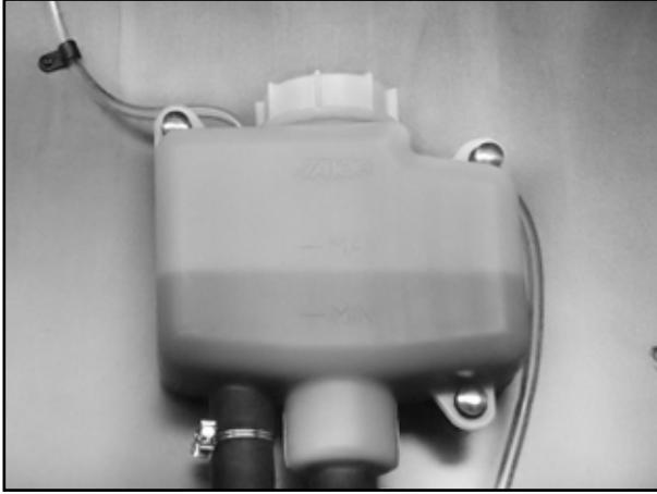
Tank for the control and refill of heating liquid
